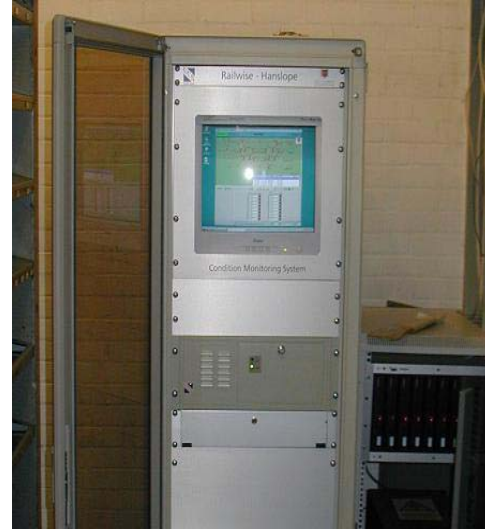
Figure 2 – Railwise RCM Track-side PC
